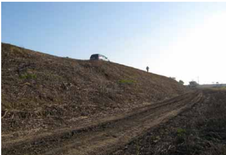
Steep landside levee slope
