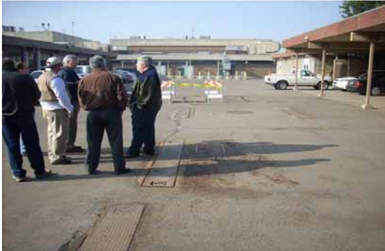
Northwest view of possible point of internal inundation from the underground effluent lines (under grates in pavement) leading into the head works
