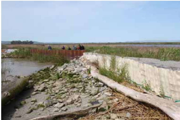
Western view of the waterside conditions along the Sacramento River. Sheet piles and a cellular wall filled with crushed gravel were installed to prevent overtopping
