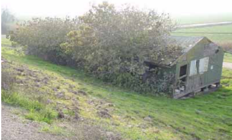
Down slope view of old historical labor camp housing at toe of levee slope
