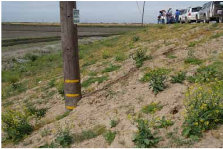
Northern view of landside conditions in repaired area Note: Surface cracks, erosion gullies at mid slope
