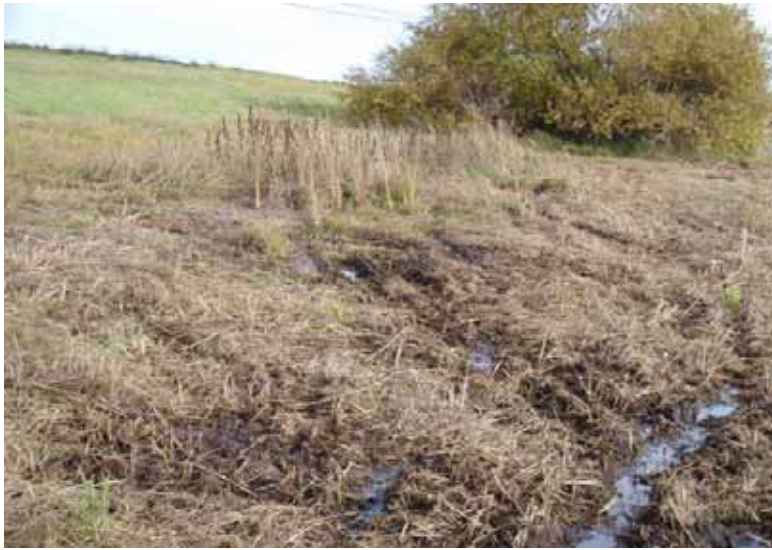
Southern view of levee slope where wet spots are noticeable and indicate seepage
