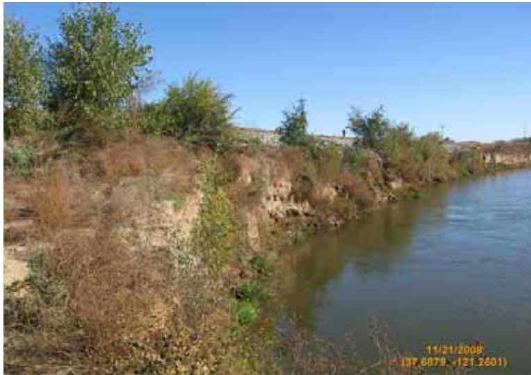
Erosion in the waterside slope
