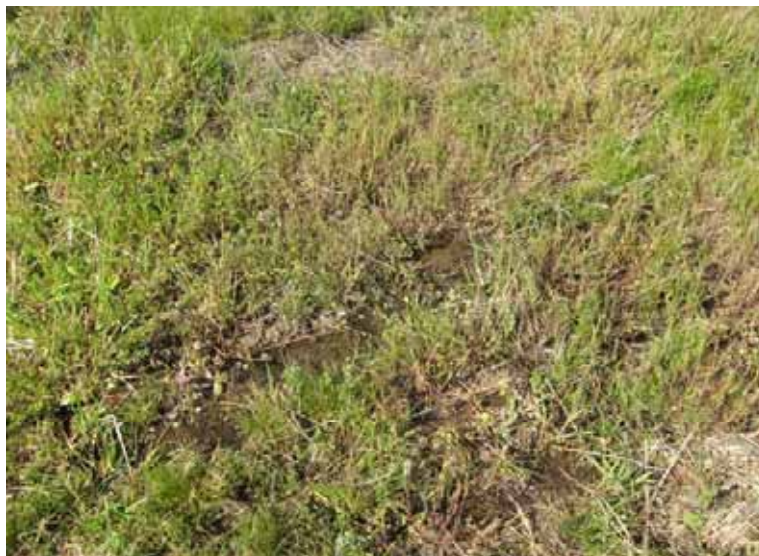
Standing water and wet ground on the landside slope as a result of seepage
