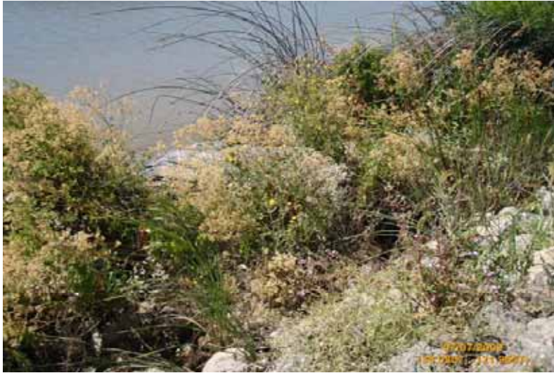
View of levee failure caused by ongoing subsidence Note: Levee was set back away from failure
