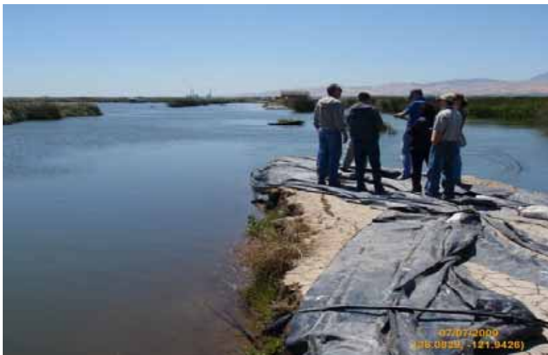
Southern view of the break in Blue Bird Road with other side of break in background (Area was repaired previously as indicated by the remaining sand bags and tarps)
