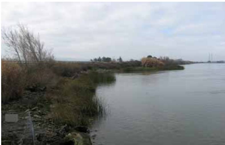
Overview of site, looking downstream from intake Heavy erosion along Sacramento River requires repair
